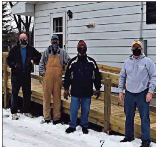
Habitat for Humanity Benzie Site Selection and Construction Committee members (from left to right) Don Bridges, Steve VanDePere, Bill Frostic and Glen Tracy, recently constructed a ramp for the widow of a WWII veteran. (Courtesy photo)
